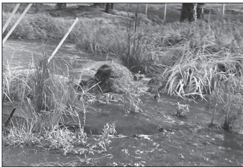
Photo shows wetland area at NE corner of the property and Oranole Way. Note the location of the silt fence (underwater) as stormwater rushing through the property, including water from a pond, releases the muddy water flowing over the hay bales, silt fence and over the pavement of Oranole Way
