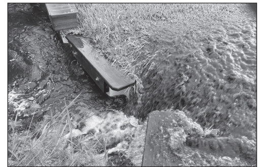
Photo shows mud gushing into the Bear Lake Canal From the August 10, 2020 rains washed out of the Construction site directly into the channel to the canal
