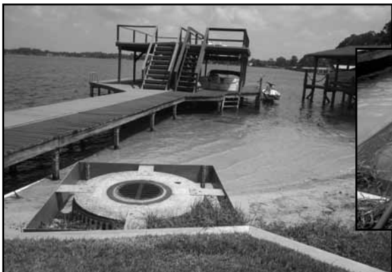
Left: Low water at outfall manhole from Bear Lake to Cub Lake.
