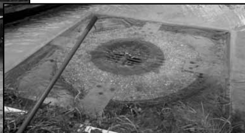
Above: High water at outfall manhole from Bear Lake to Cub Lake.
