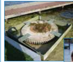
Barrier put around manhole by Seminole County.
